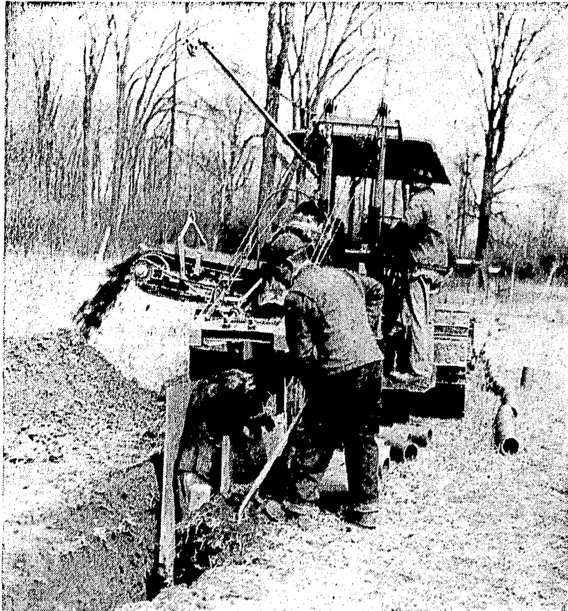
INCREASING farming efficiency by the installation of a complete tile drainage system on the Gerald Eifert farm on Willoughby road in Alameda township was the result of this operation. Russell Dowling, drainage contractor, is controlling the depth of the trench by sighting over the targets. The man in the trench is putting the tile in place. And Eifert, with shovel, is blinding the tile with loose topsoil. This crew can install as much as 20 rods a day.
